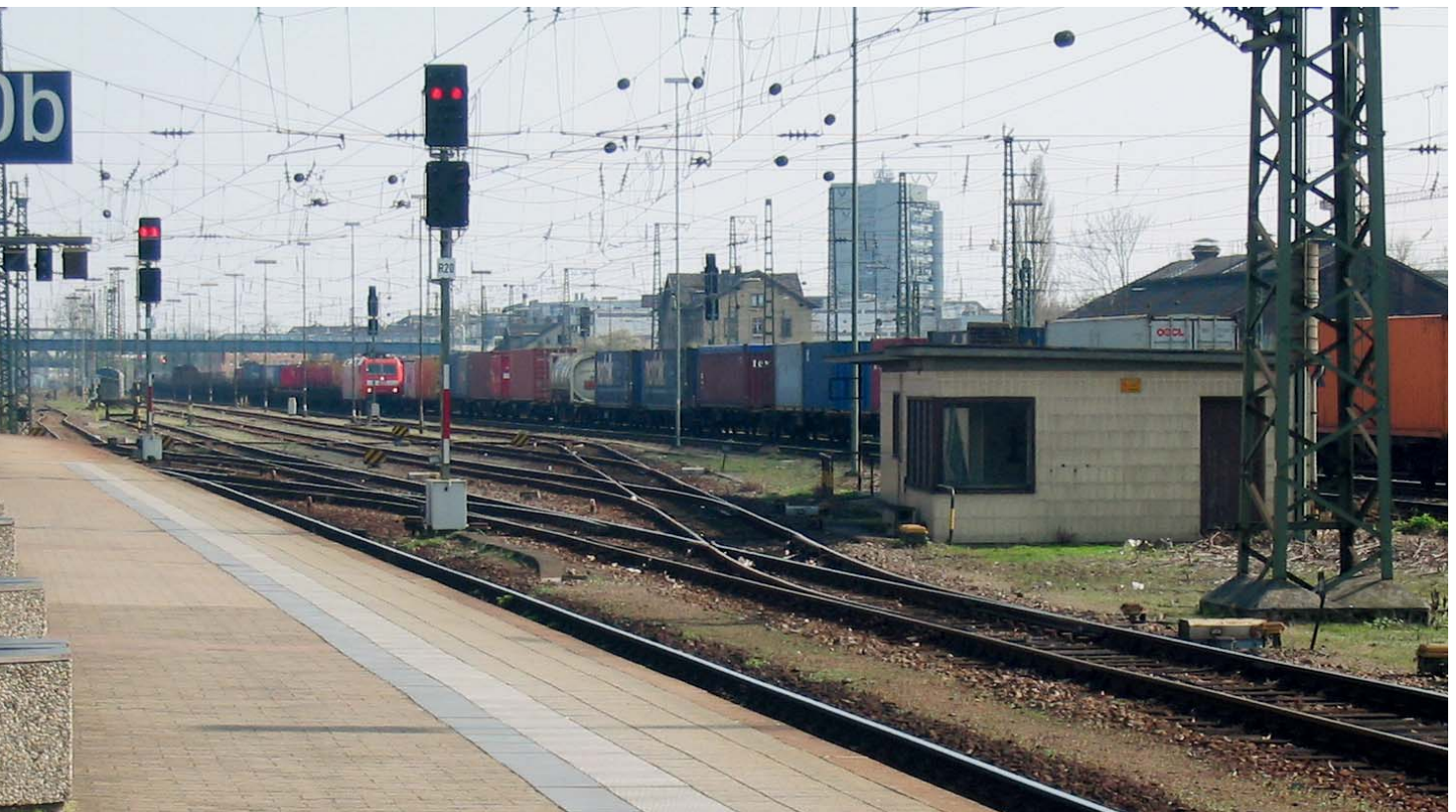
Figure 1: 15 kV overhead contact line near points in Mannheim railway station
