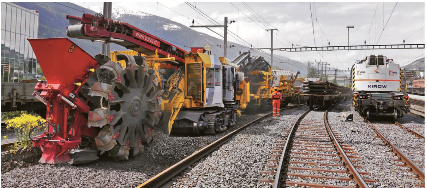
Construction site for switch replacement with excavator: walking-floor bulk freight wagon with screen and 'Reiner' crawler chassis (background on the left), flat wagon for yoke transport (background in the middle on the right) and rail crane for discharging switches (on the right)
