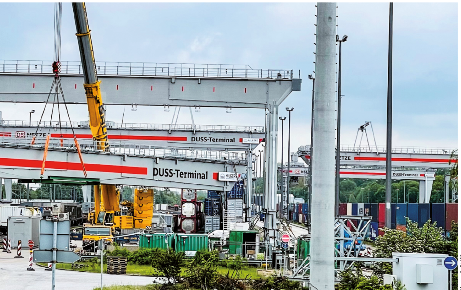
DUSS Terminal Hamburg Billwerder: Crane beam modernisation completed by the end of 2021.
